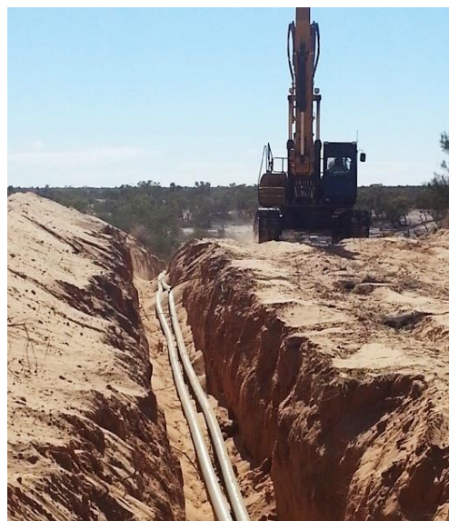
Connecting Spitfire oil field to the Growler Bulk Storage Facility
